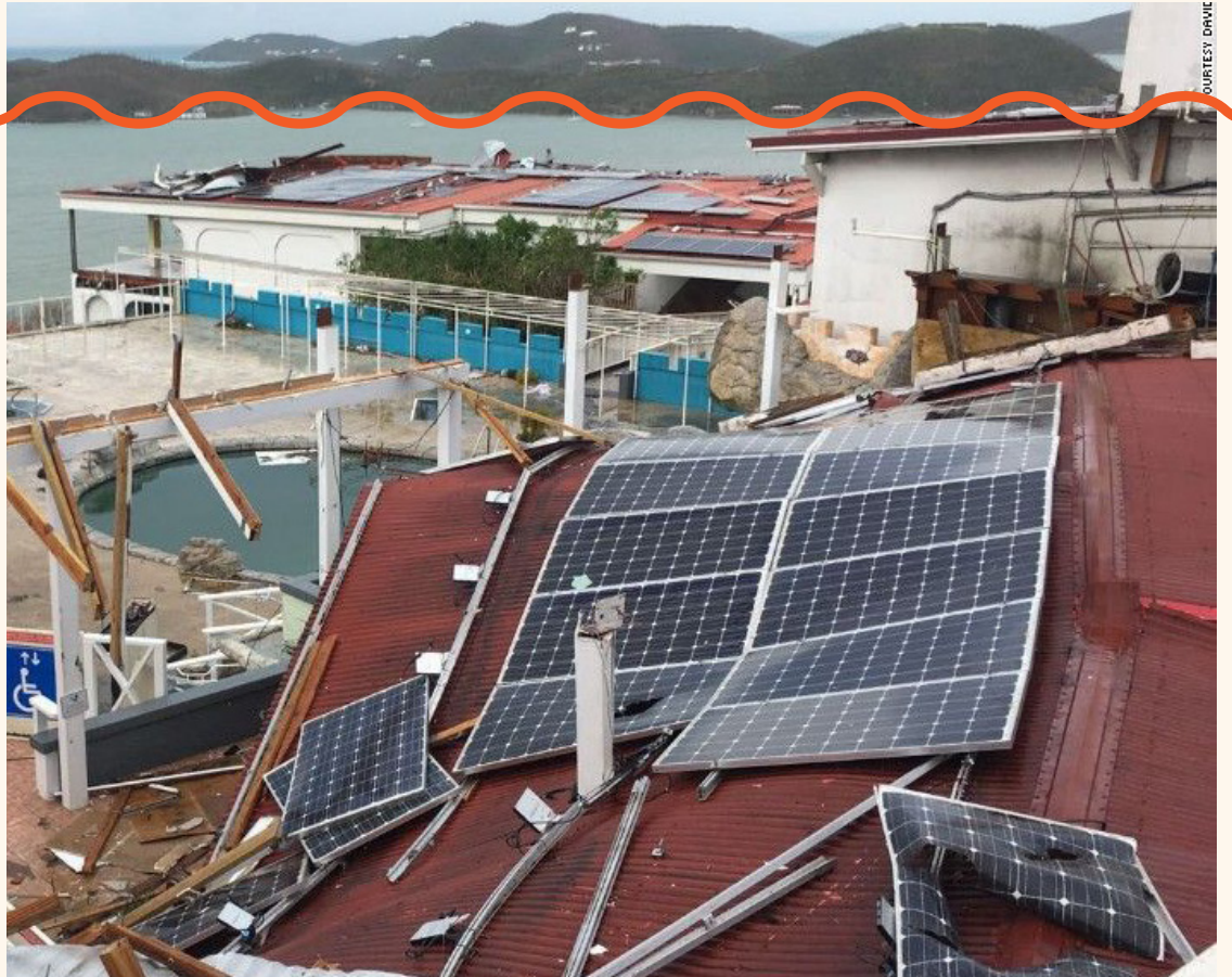
Building after 2017 Storms, Source: CNN
